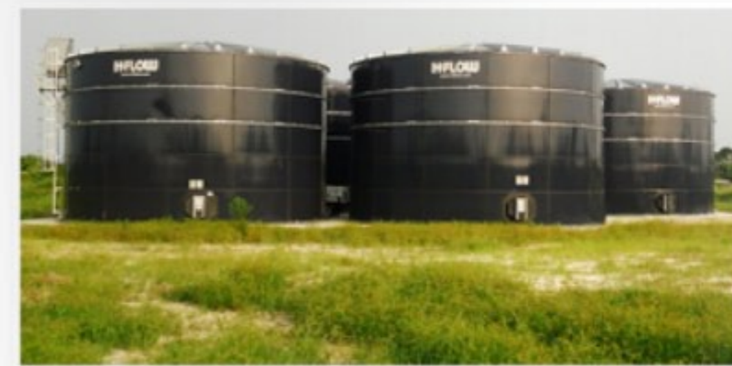
The plant consists of a sequencing batch reactor in four large glass-fused-to-steel tanks.
